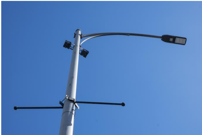
City Surface Lot Camera Sensors powered from base of luminary
