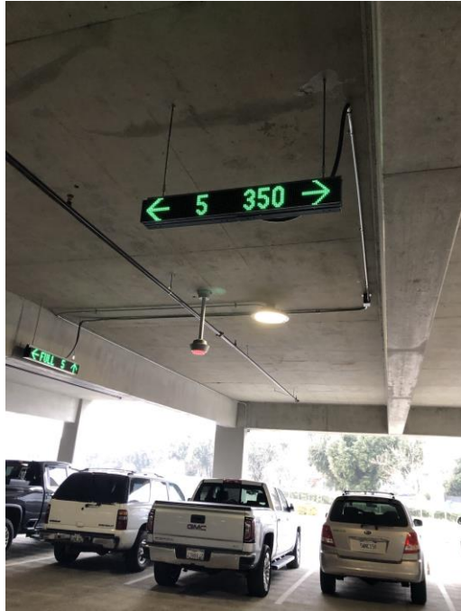
Airport Garage: Pre-embedded, examples of junction box misplacement
